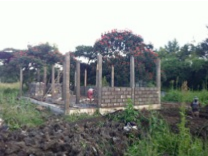
Start of the walls of the MWH and the foundation of the kitchen
