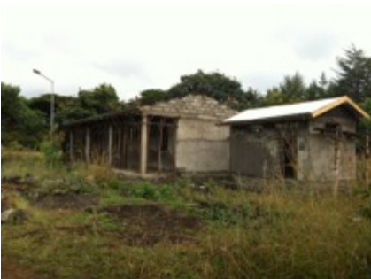
Current building status: the roof of the MWH and kitchen are almost finished
